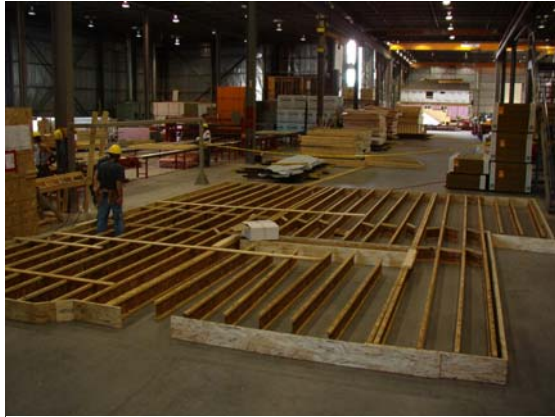
Mattamy Homes' Stelumar division builds panelized floors using iLevel® Nextphase®-JobPack precision-cut and labeled products.
