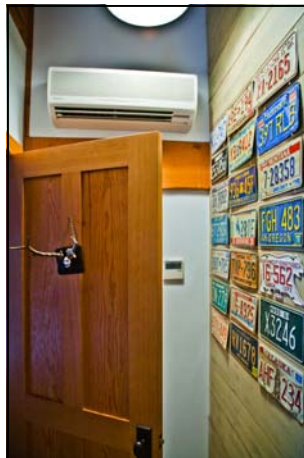
Daikin installed 2 RXYMQ VRV-S outdoor units, 3 FXAQ wall mounted units and 3 FXDQ slim-duct built-in concealed ceiling units and 1 FXSQ.
