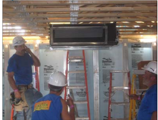
The FXSQ Concealed Ceiling Unit being installed in the Hill's new home.
